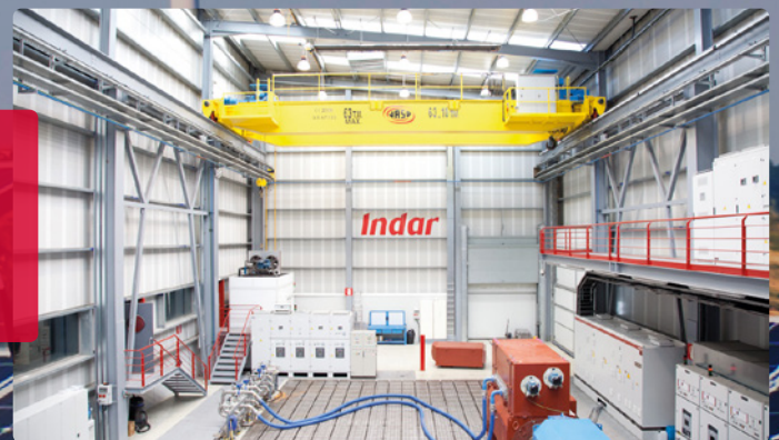
Beasain (Gipuzkoa) Rotating electric machines laboratory
