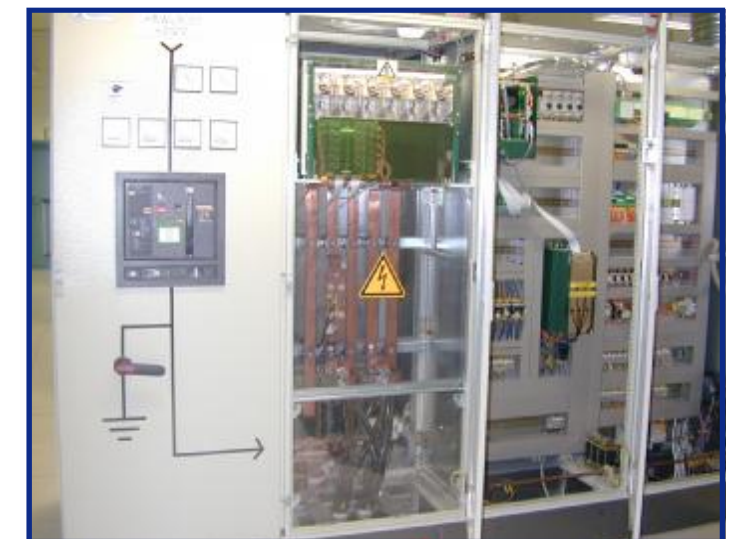
DC Motor Control Center
