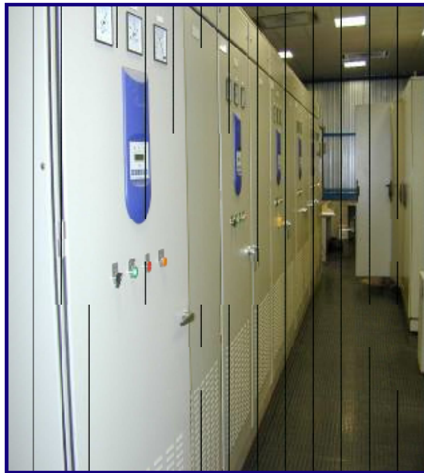
VVVF Motor Control Center
