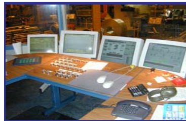
Main Control Pulpit
