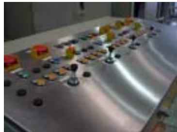
Main Control Pulpit
