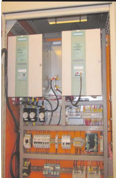
12 pulse converter system
