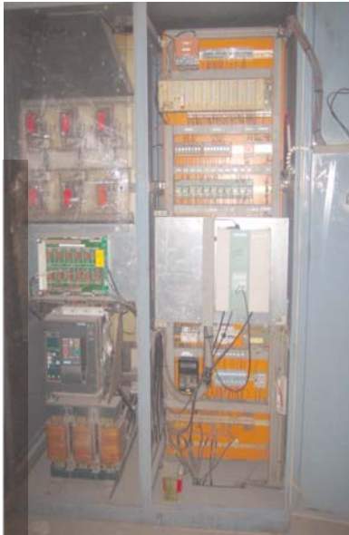
6 pulse converter system
