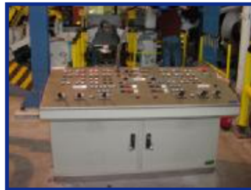
Uncoiler Local Panel
