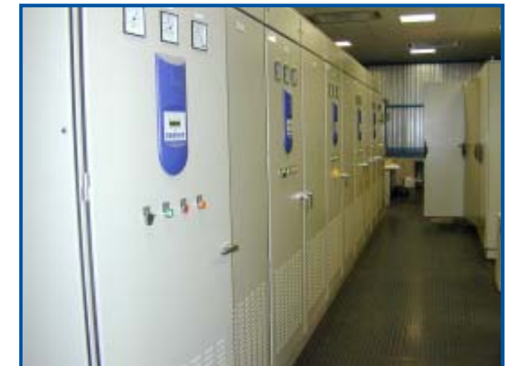
DC-Motor Control Center
