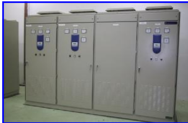
DC Motor Control Center
