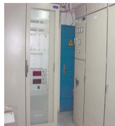
Auxiliary drives and electrode Control Equipment
