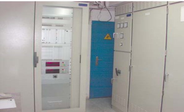
Furnace Regulation Equipment
