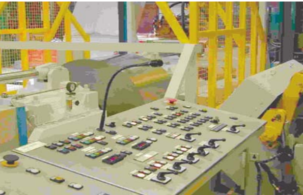
Furnace Main Pulpit
