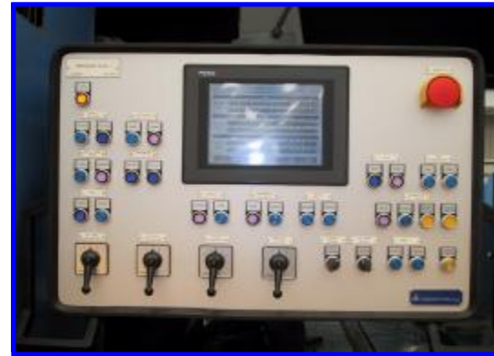
Local Control Panel
