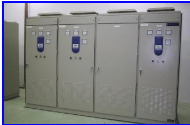
DC Motor Control Center
