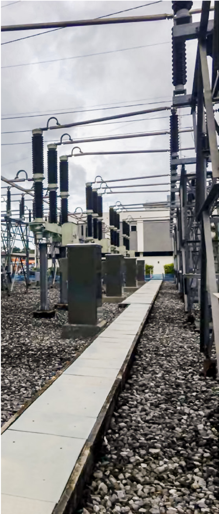
Fiber optic channeling of the process bus
