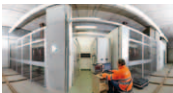
METRO BILBAO INGEBER energy recovery system: 5 units.
