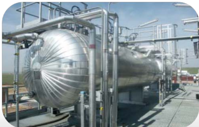
CAPARROSO - Biodiesel Plant
