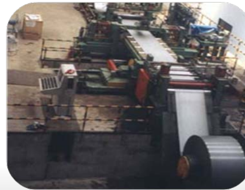
Pickling Line ARCELORMITTAL
