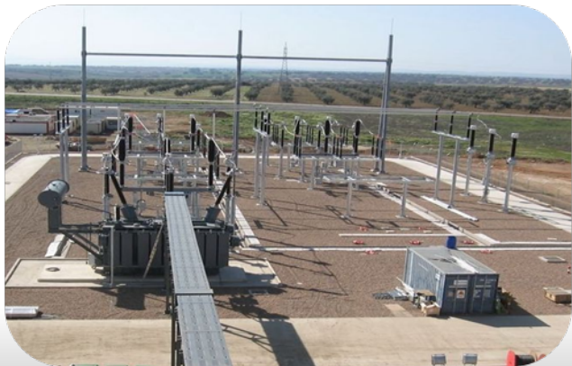
LA RISCA Substation
