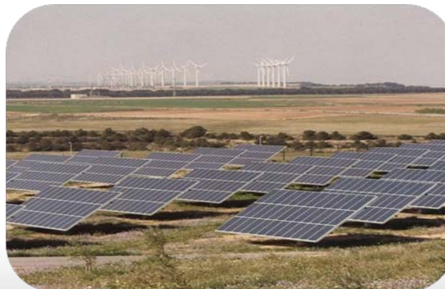
CASTEJÓN - Photovoltaic plant
