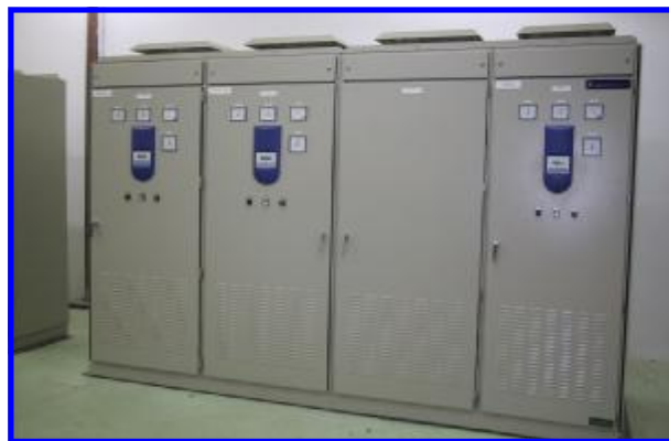
DC Motor Control Center
