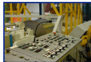
Tension reel - Local control desk
